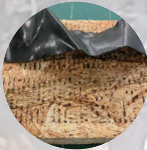
Completely Peeled Off
