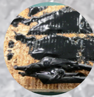
Completely Peeled Off
